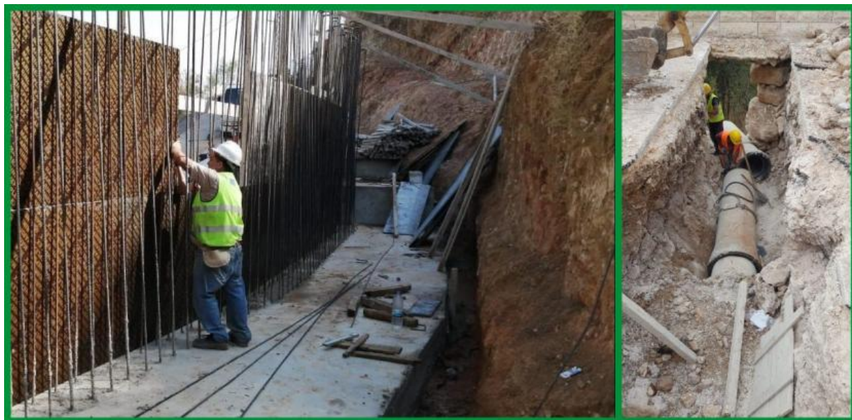
CSP carries out construction works on the Markebta retaining wall (left) and the irrigation piping in Kfar Hilda (right).
