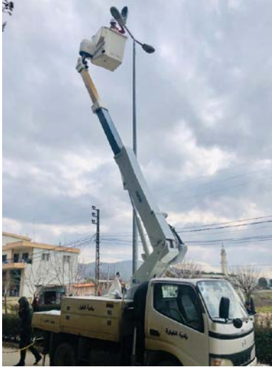
CSP installs streeting lighting to reduce tensions in El Khiara by bolstering residents' sense of safety and security.
