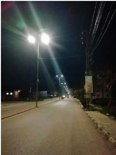
The CSP-provided street lighting in El Khiara
