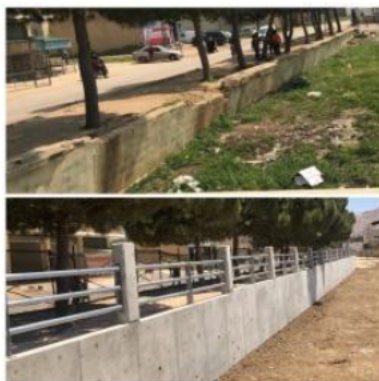
The Ghazze retaining wall before and after CSP's rehabilitation project LEBANON COMMUNITY SUPPORT PROGRAM
