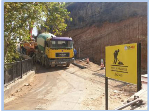
CSP constructs a section of a 70-meter long, 3-meter high retention wall to prevent soil erosion at the main entrance of the village of Markebta (North). The wall will reduce the tensions among about 6,000 residents by reducing public safety risk and the possibility that a landslide would force the closure of the main road connecting the village to the surrounding area.
