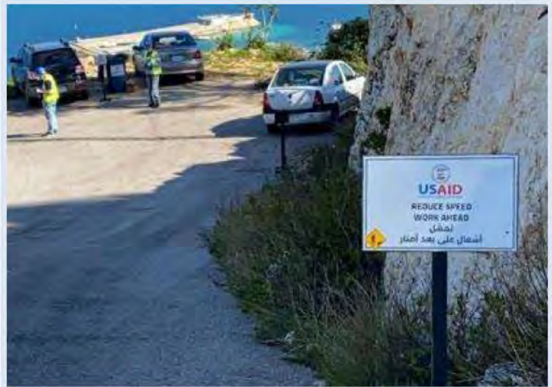
USAID safety road sign installed at the labor-intensive work site in the northern village of Dedde.
