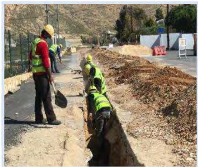
Excavation work in Ras Baalbek (Beqaa) to enhance the village's irrigation system and support underserved farmers.
