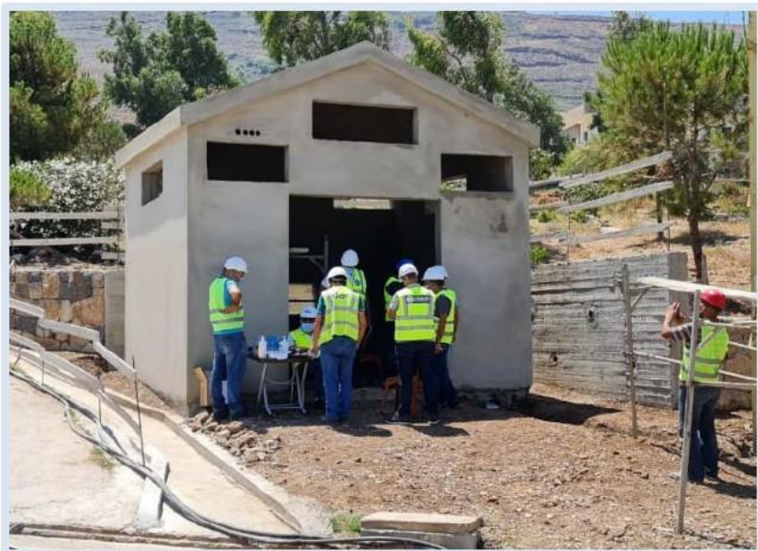
Photo of the newly constructed electrical transformer room in Khirbet during a site visit conducted by CSP, its local subcontractor and USAID's partner CDM Smith.
