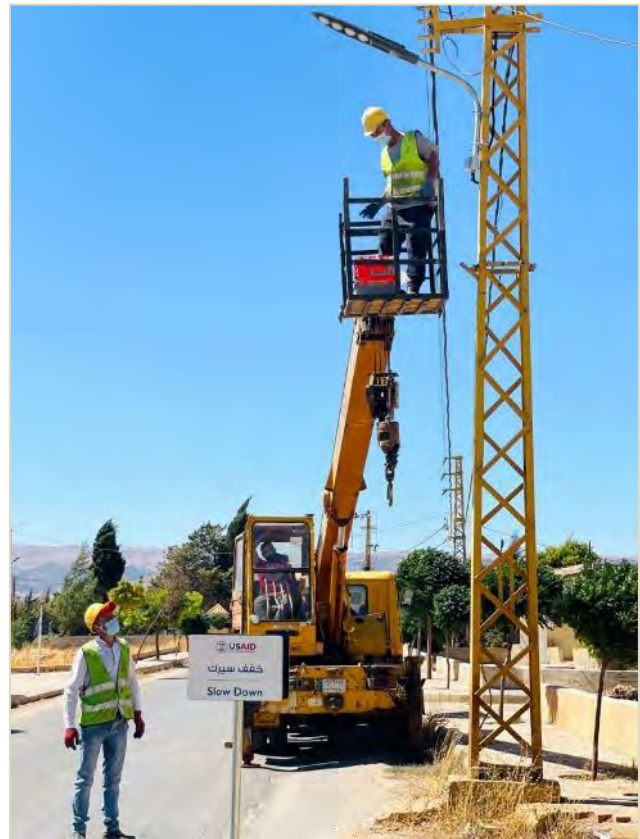
UASID/CSP workers install new LED streetlights in strategic locations in Hawch Barada (Beqaa)
