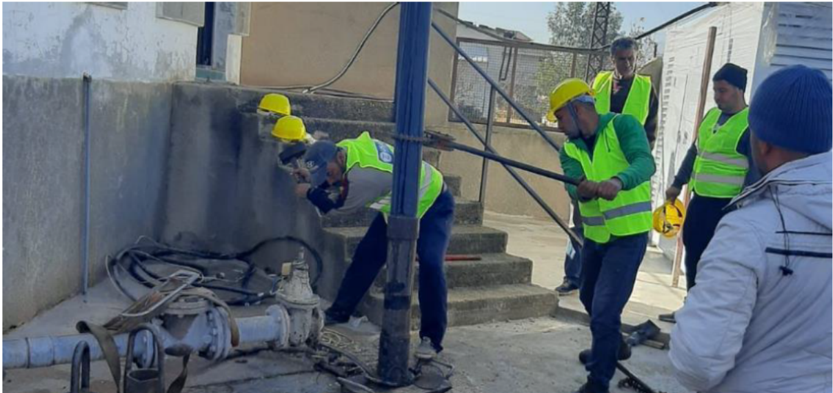
USAID/CSP site work in progress in Sultan Yaacoub to ensure sustainable, solar-powered energy for the Loussiya water pump – December 2021
