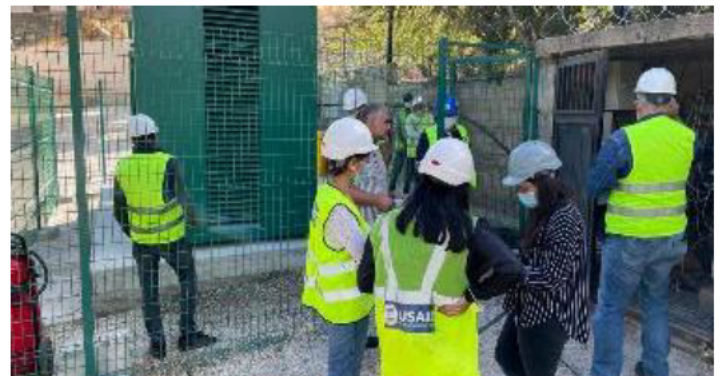
USAID/CSP inspection visit to Aaiha, where CSP provided and installed a backup generator to ensure power supply – Beqaa
