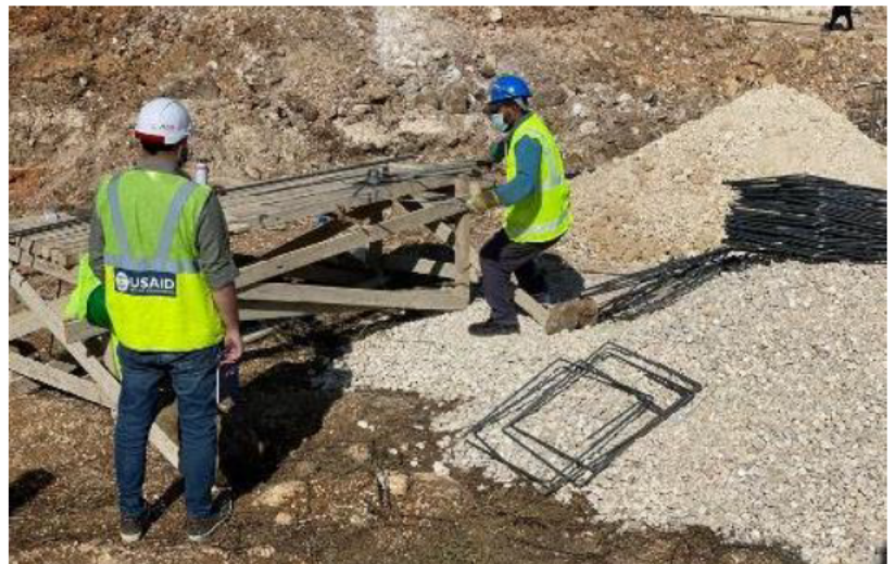
USAID/CSP contractor mobilizes for site preparations in Hasbaiya for the installation of solar panels to ensure electricity provision – South Lebanon
