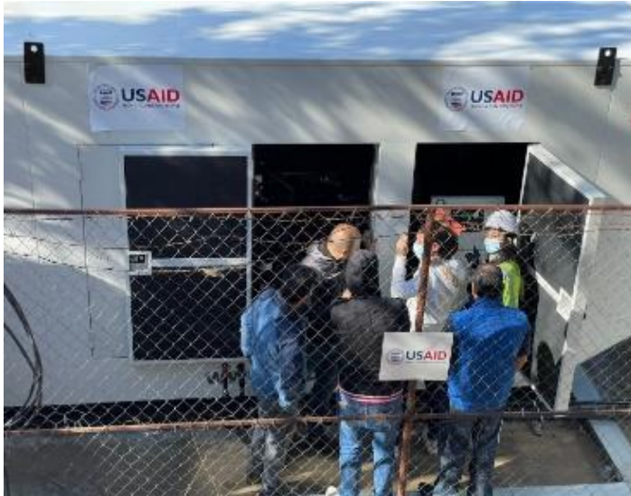
USAID/CSP inspects its provided and installed backup generator on site in Dahr el Ahmar - Beqaa
