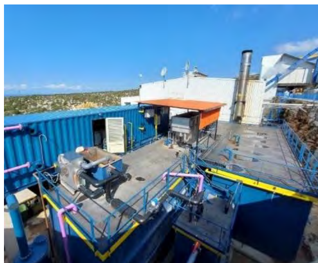
CSP/USAID site visit to Cortas Industrial Treatment Plant, Jbeil – February 2022
