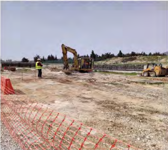
CSP initiates grading and earthwork in preparation for the Aaitanit WWTP rehabilitation and sludge management upgrade.
