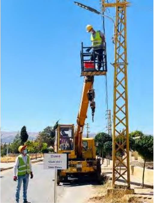
CSP installs LED-type streetlights to enhance safety and security in Hawch Barada (Beqaa)
