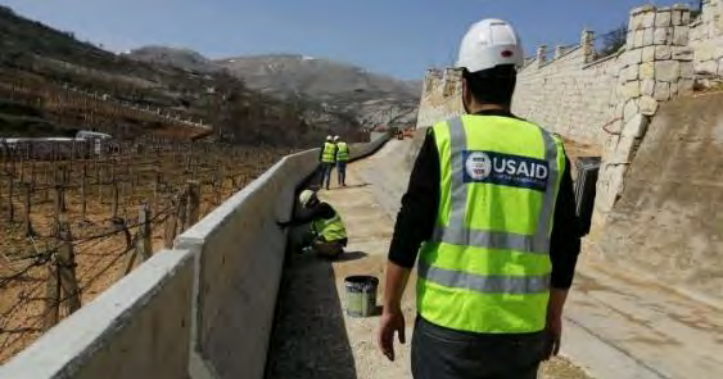
Ongoing works in Nabi Ayla to construct a retaining wall and side rails to enhance public safety (Beqaa)
