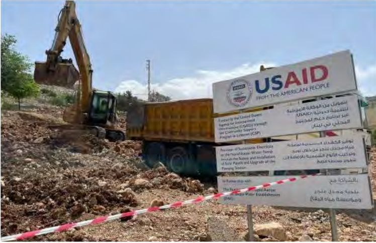
USAID/CSP ongoing works in Majdel Anjar to ensure continuous energy to water pumps through solar solutions
