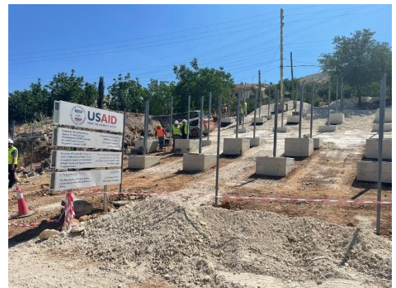
USAID/CSP ongoing works in Majdel Anjar to ensure continuous energy to water pumps through solar solutions
