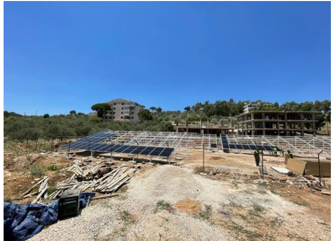
USAID/CSP ongoing works in Hasbaiya to supply and install on-grid solar farms
