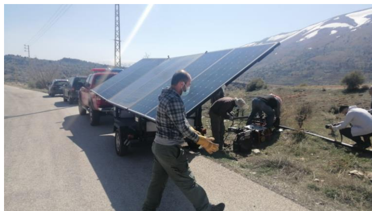
Ainata el Arz farmers utilize CSP's provided solar welding machine to repair irrigation pipes
