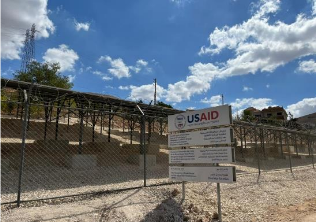
Photo of the site in Majdel Aanjar, where CSP installed solar panels to ensure operation of the water pumping system (Beqaa)
