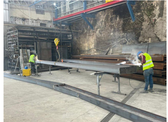
Works on the roof of the upgraded drying bed at the steel manufacturer
