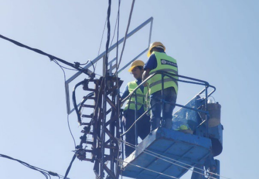
CSP completes the delivery and installation of 100 solar streetlights on existing poles to improve safety and security in Kfar Jarra
