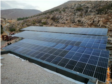
Photo of the site in Es Soutan Yaaqoub, where CSP installed a solar farm to ensure the operation of the water pumping system
