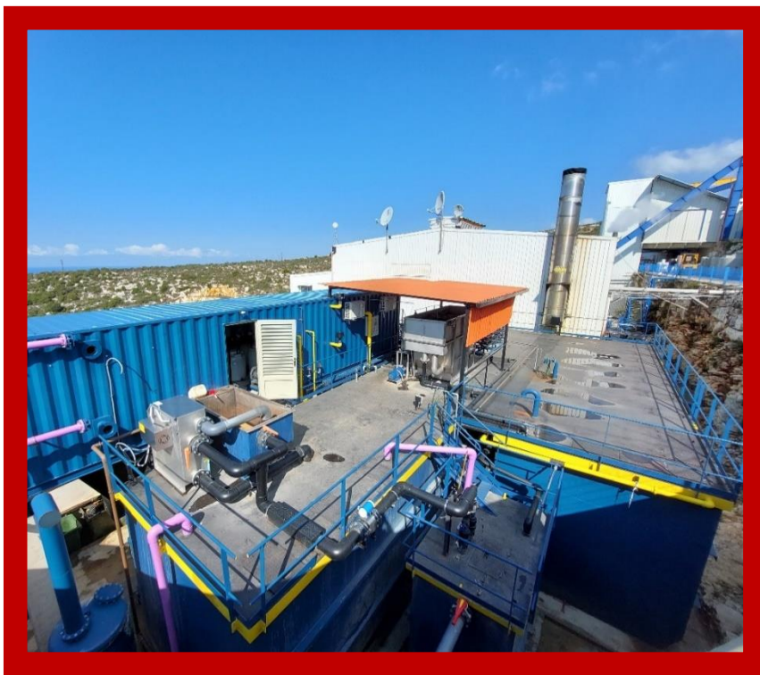
Industrial wastewater treatment plant in operation at Cortas' factory – February 2023
