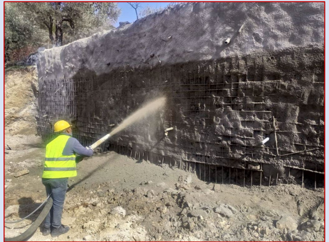
CSP shores concrete during construction of the USAID-funded Bchaale wastewater treatment plant
