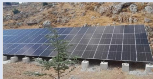
Solar farm works in Tannoura, Beqaa, implemented by the municipality to ensure water supply to residents. The project is funded by community members following support from CSP in proposal writing, raising more than $85,000 – Aug 2023
