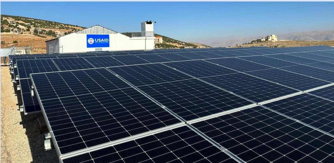
The USAID/CSP upgraded water pumping station in Bechwat, Beqaa – Nov 2023
